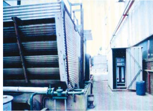
Ozone cooling Tower in Operation
