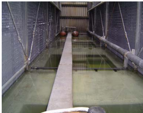
Tower Sump after Ozonation
